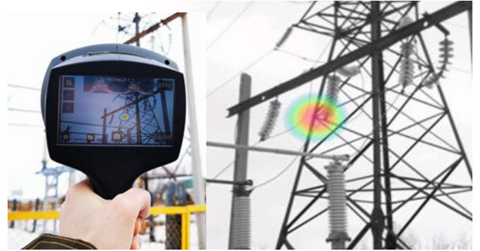
Image 1. The NL Camera found a surface discharge on one of the insulators in the garland of insulators VL 110 kV. The partial discharge was missed by the infrared and UV cameras.
